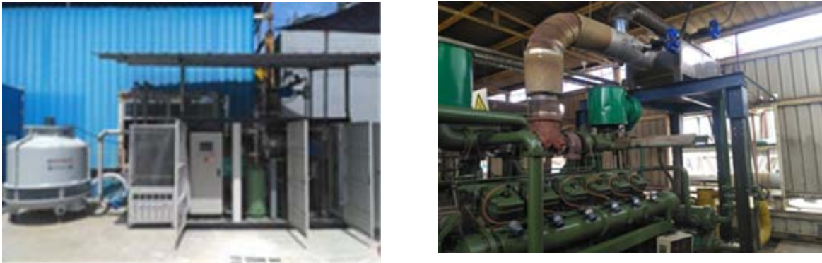
Fig.10: ORC demonstration projects from Coalbed gas Engine waste heat
