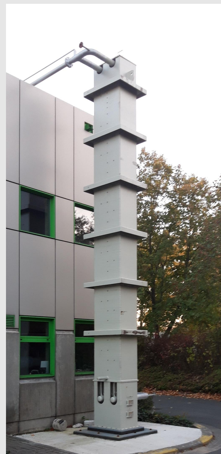
Figure 3. Picture of the installed shell and tube LHTES (campus Kortrijk Ghent University).
